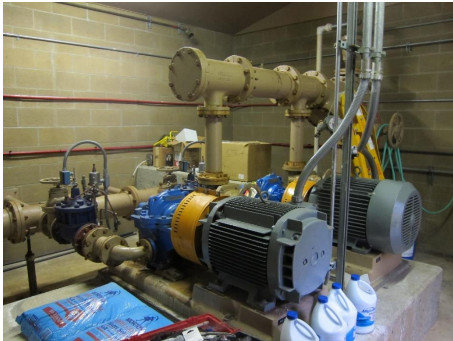
North Bank BPS (Inside)
