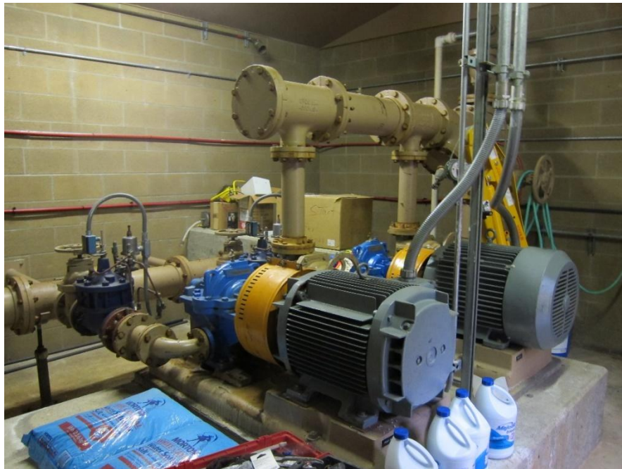
North Bank BPS (Inside)
