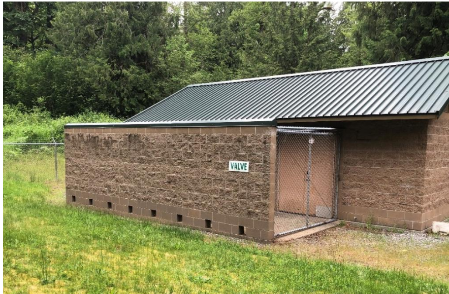
North Bank BPS (Outside)
