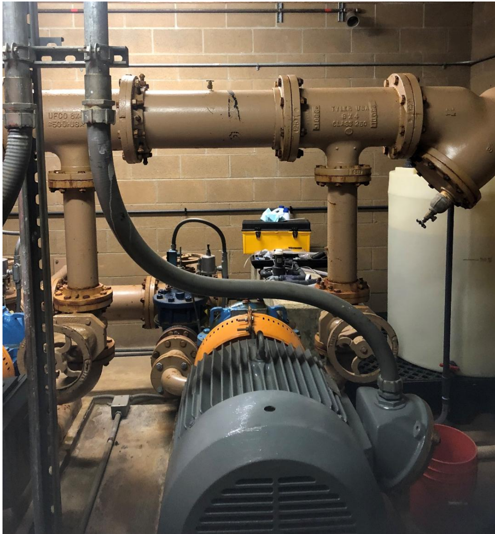
North Bank Pump Station
