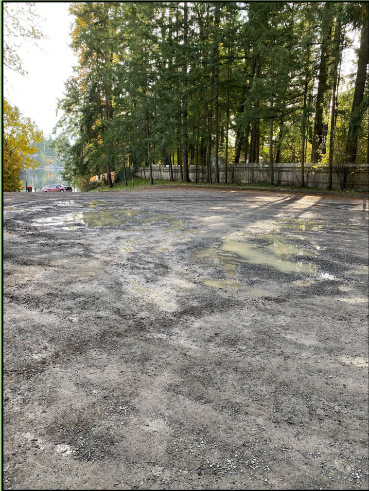
Pothole conditions at the Lake Sawyer Boat Launch parking lot.
